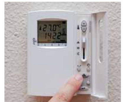
Install air conditioner controls to allow timing and temperature regulation, to minimise energy consumption.
